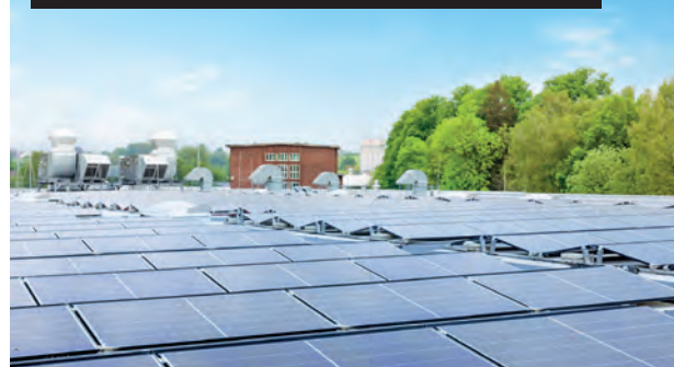
Photovoltaic system at the Wipperfürth plant
